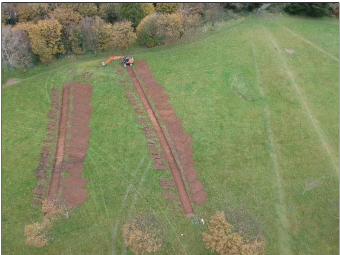
Plate 43: Aerial of T8 (right) and T9 (left) facing north
