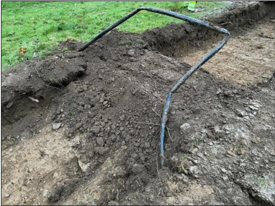
Plate 7: View of modern service pipe within the topsoil matrix of T1
